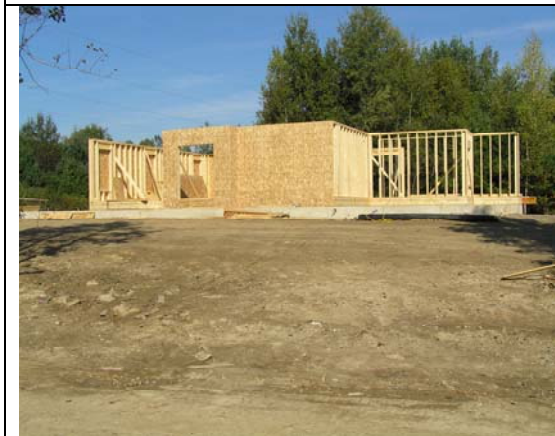
Figure 15. The Builder's Longkill subdivision in the Town of Ballston. New home with backfill.
