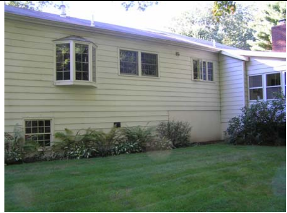
Figure 2. Our backyard showing raised basement. The basement was built above ground and backfilled.
