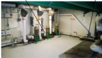
Condensate return tank (right side of image)
