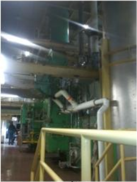
Front Profile of Existing Boilers
