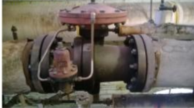
Pressure Reducing Valve (PRV)
