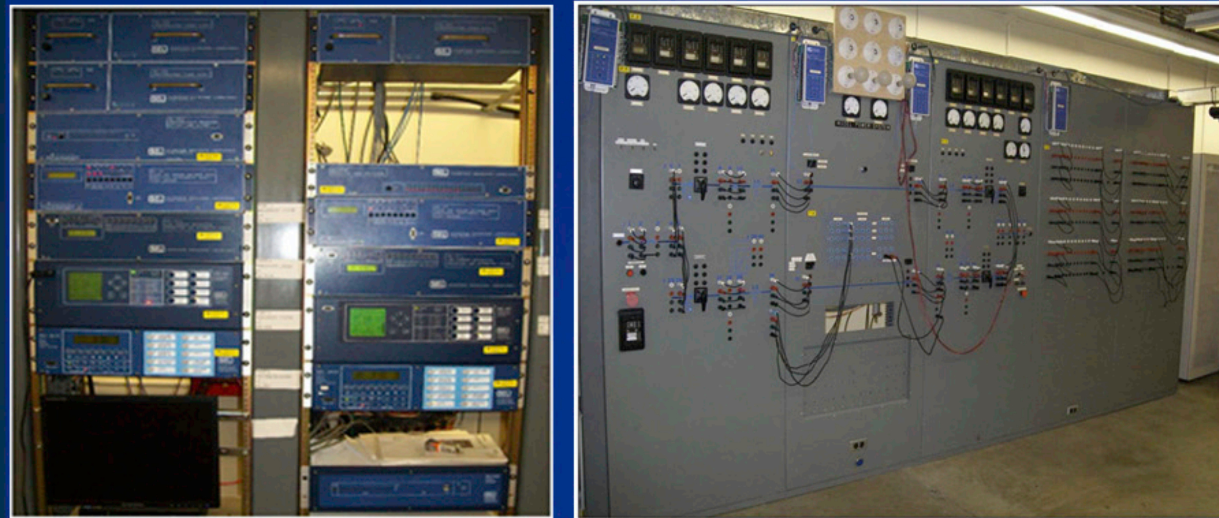
Old Relay Rack
