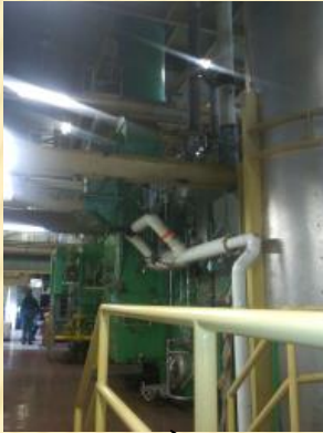
Front Profile of Existing Boilers
