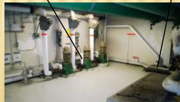
Condensate return tank (right side of image)
