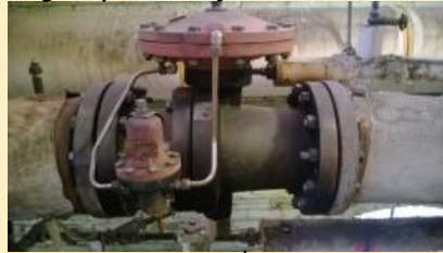
Pressure Reducing Valve (PRV)
