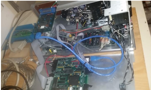
Figure 1. Old Control Electronics
