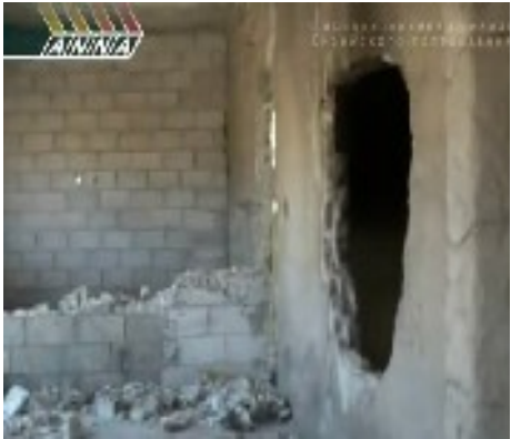
Horizontal “shelling” damage to a home, from ANNA News, May 26
